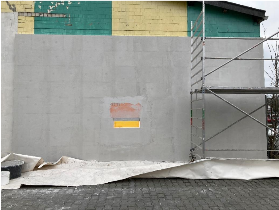
Figure 25: Test façade with completed reinforcement layer (base coat) with block-out for an EPS window
