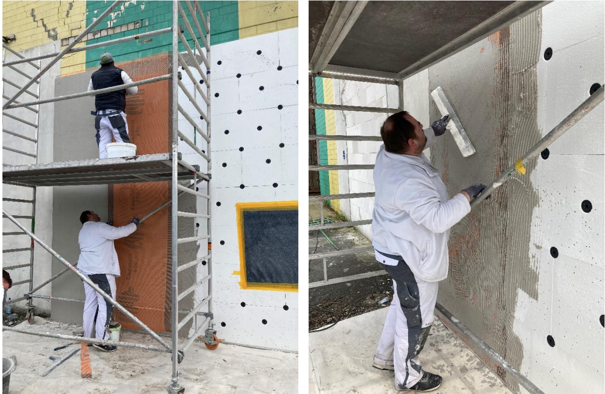
Figure 24: Reinforcement mesh is attached (left) and incorporated (right) into the base coat layer
