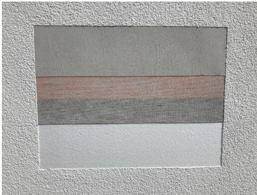
Figure 29: Close up of window for the CREAToR EPS including build-up of layers
